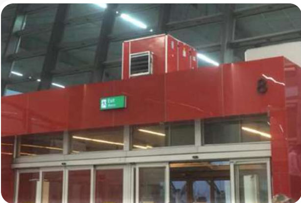
Air Handling Unit
